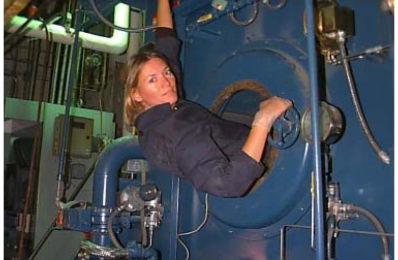
Liza Fraser exits a steam boiler during an internal inspection for a client in New York. Ms. Fraser, a regional manager, has worked at Barclay for eight years
